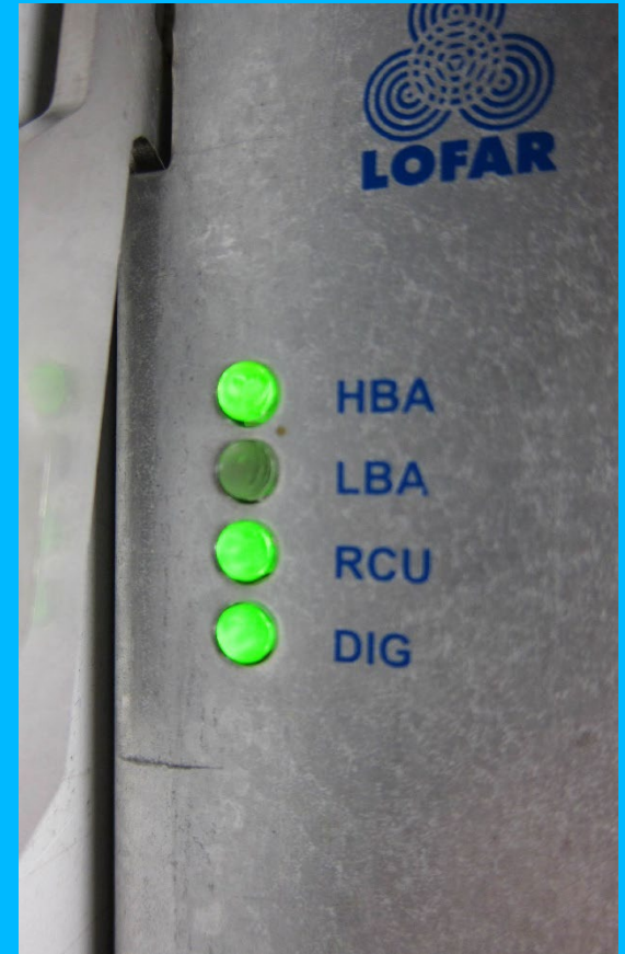
SPU with old 8 Volt power module
